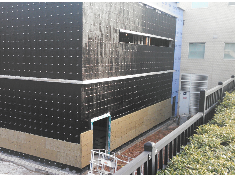
Tremco’s ExoAir® 220 Fluid-Applied Vapor-Permeable Air Barrier Membrane has been applied to the wall of the extension and ExoAir® 110 Self-Adhered Air and Vapor Membrane at the door opening. The brick tie bases have been installed, and SECO has started installing the mineral wool insulation.
